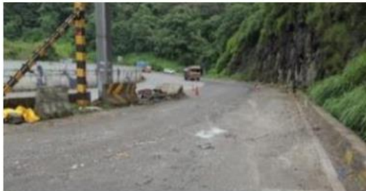
FIGURE 11: A SHARP CURVE AT KHOPOLI EXIT WHICH IS PRONE TO ACCIDENTS.
