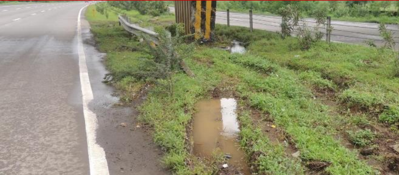
Guardrail run-out length too short
