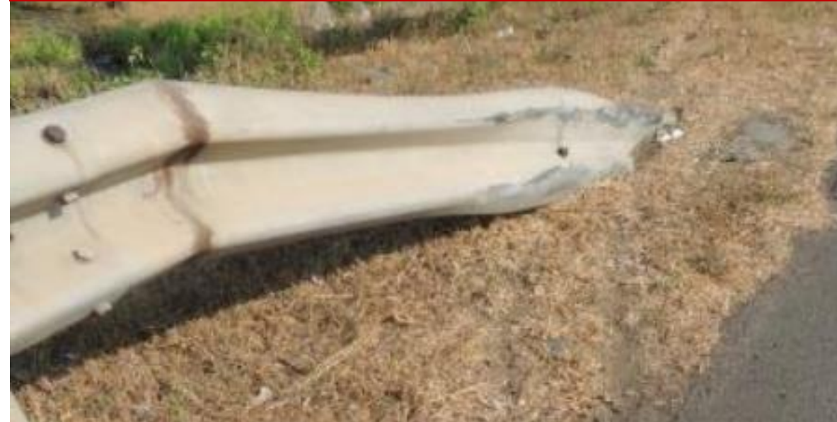
Guardrail-end tapers can launch a speeding vehicle into air
