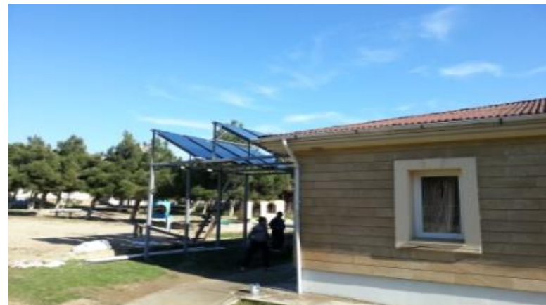
Children school SOS (20 KW electric, 44 KW heating)
