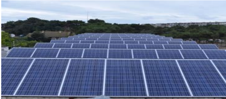
Secondary school № 235 (25KW electric, 40KW heating)
