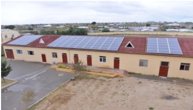
Boarding school in Turkan (25 KW electric)
