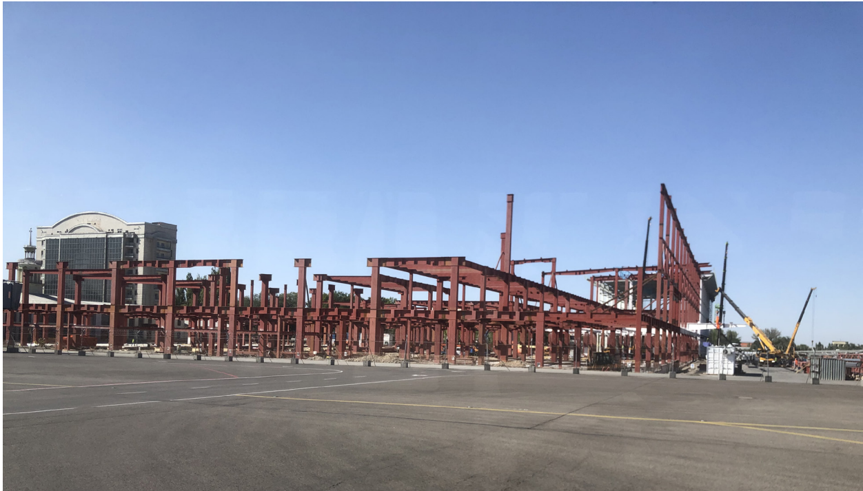
A new international terminal is under construction at Almaty Airport, which is expected to open in 2024 and increase the airport's capacity to 14 million passengers per year (photo by Brendan Sobie).
