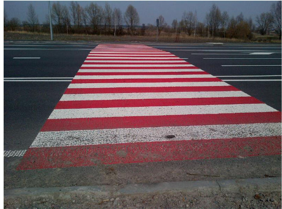
Unsafe pedestrian crossings
