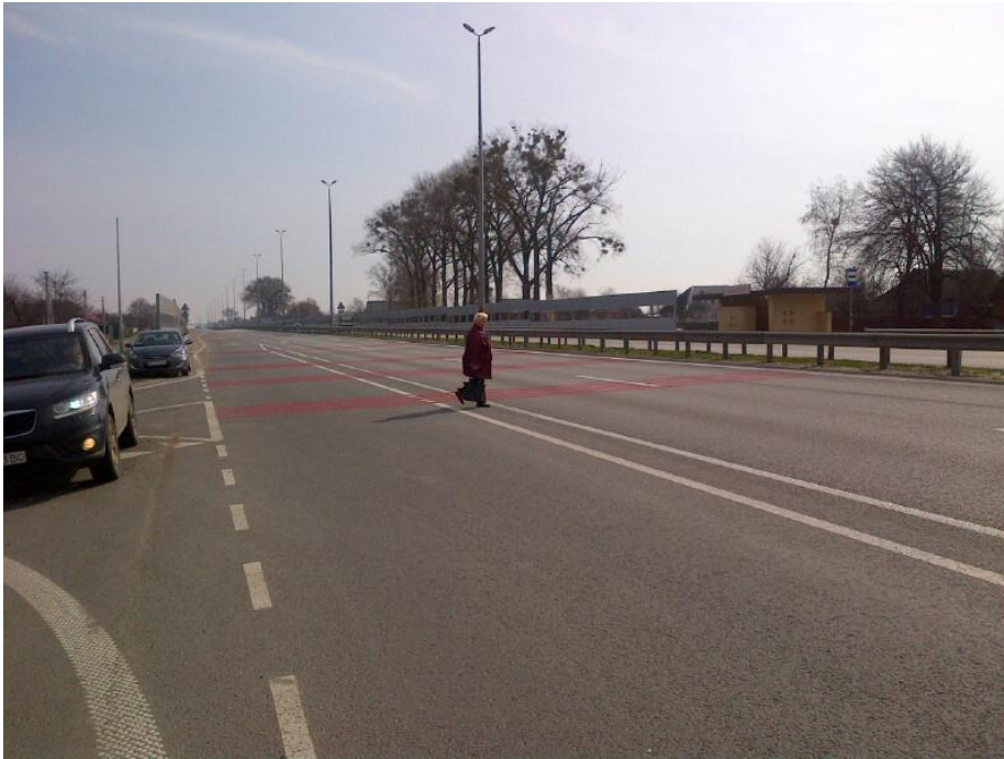
Lack of facilities for pedestrians and other vulnerable road users
