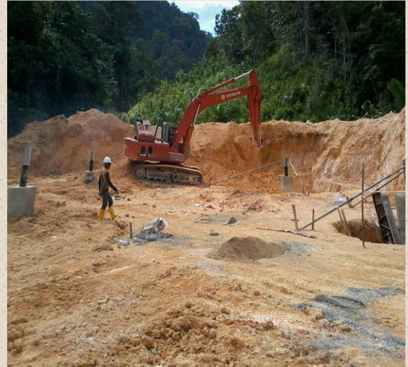
Overview of completed foundation work and backfilling in the progress at bau area kpg krokong
