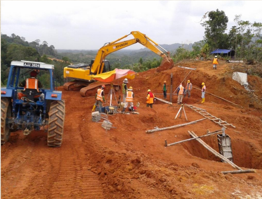
Overview of foundation work in the progress tower T14C/1 at kpg serikin
