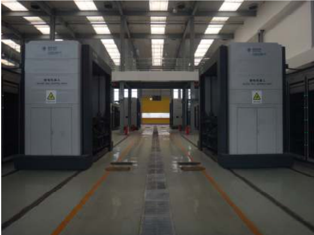
Battery swap workshop of Sihui Battery Charging and Swap Station
