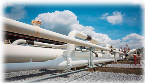
Via existing pipeline infrastructure
