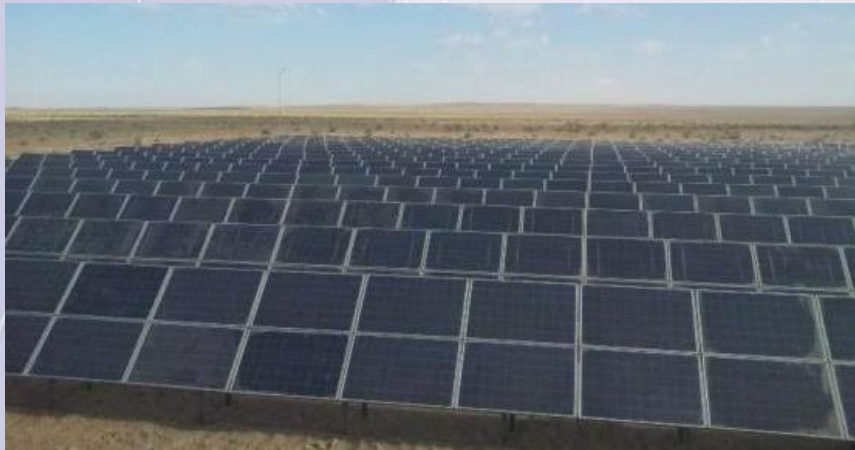
418 kW solar power station commissioned in 2013 in Zhanakorgan village, Kyzylorda Region
