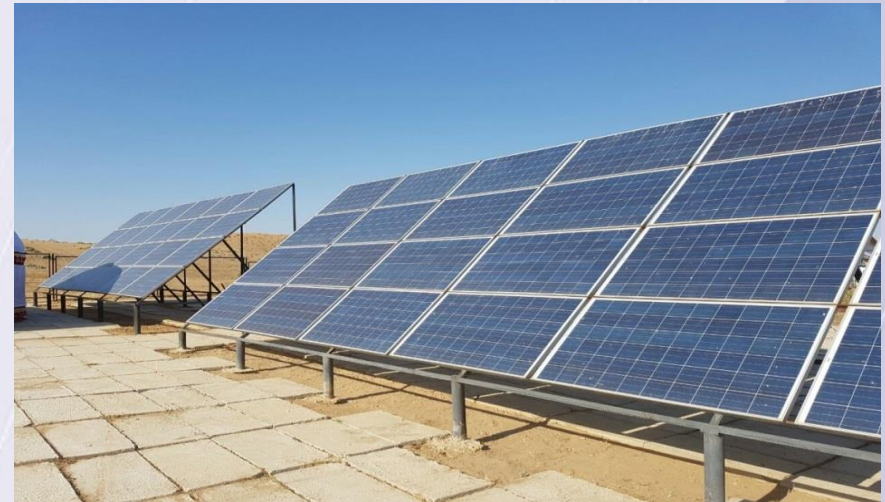
Hydrotechnical structures of pasture watering, Zhambyl region, 10 kW
