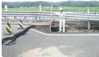
Disaster management Demolished road by an earthquake
