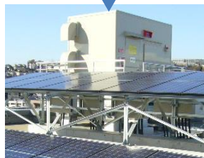
Storage battery for plants
