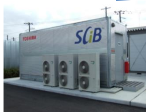
Large-scale storage batteries installed in TEPCO's Tsunashima Substation
