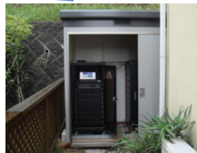
Storage battery for households
