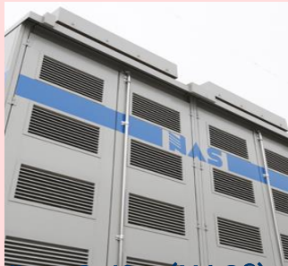
Sodium Sulfur (NAS) ® Battery System
