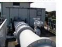
The City of Kitakyushu Waterworks Bureau's Tonda Power Station
